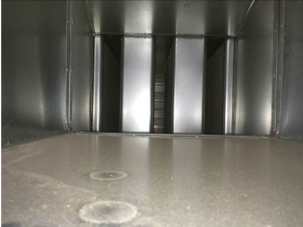
AHU BEFORE CLEANING
