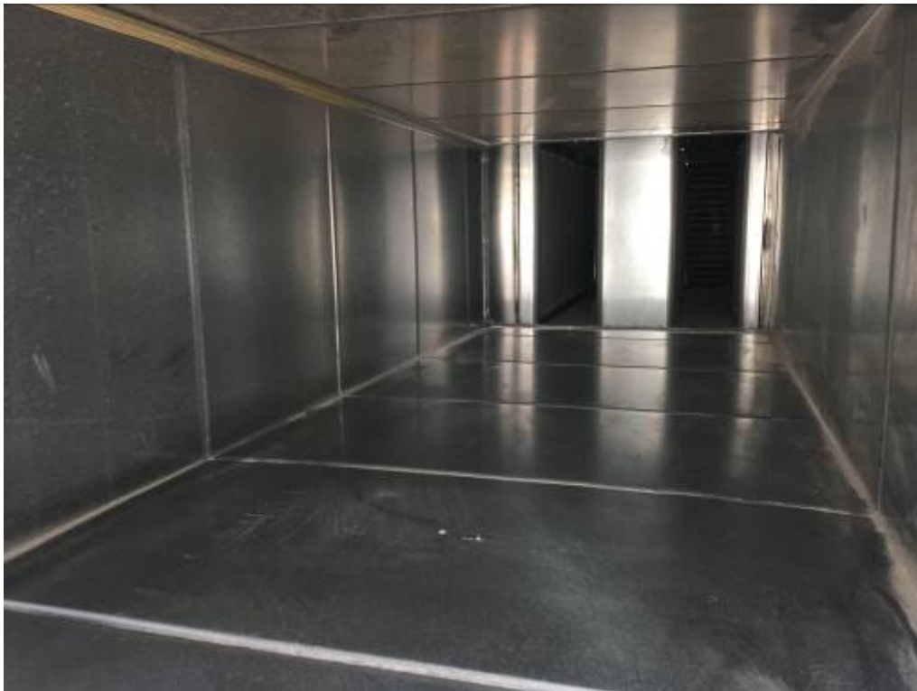
AHU AFTER CLEANING
