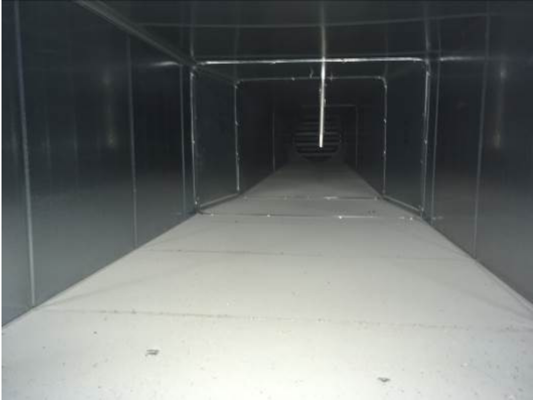
DUCTWORK BEFORE CLEANING
