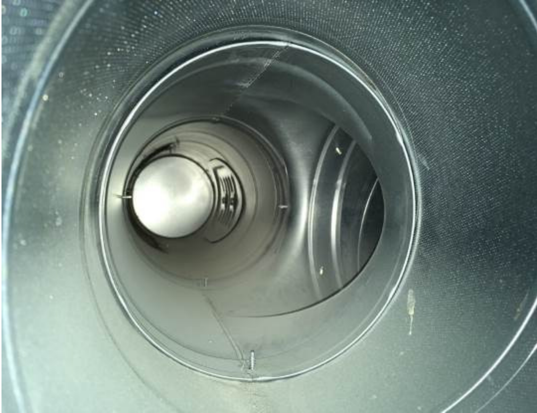
DUCTWORK BEFORE CLEANING
