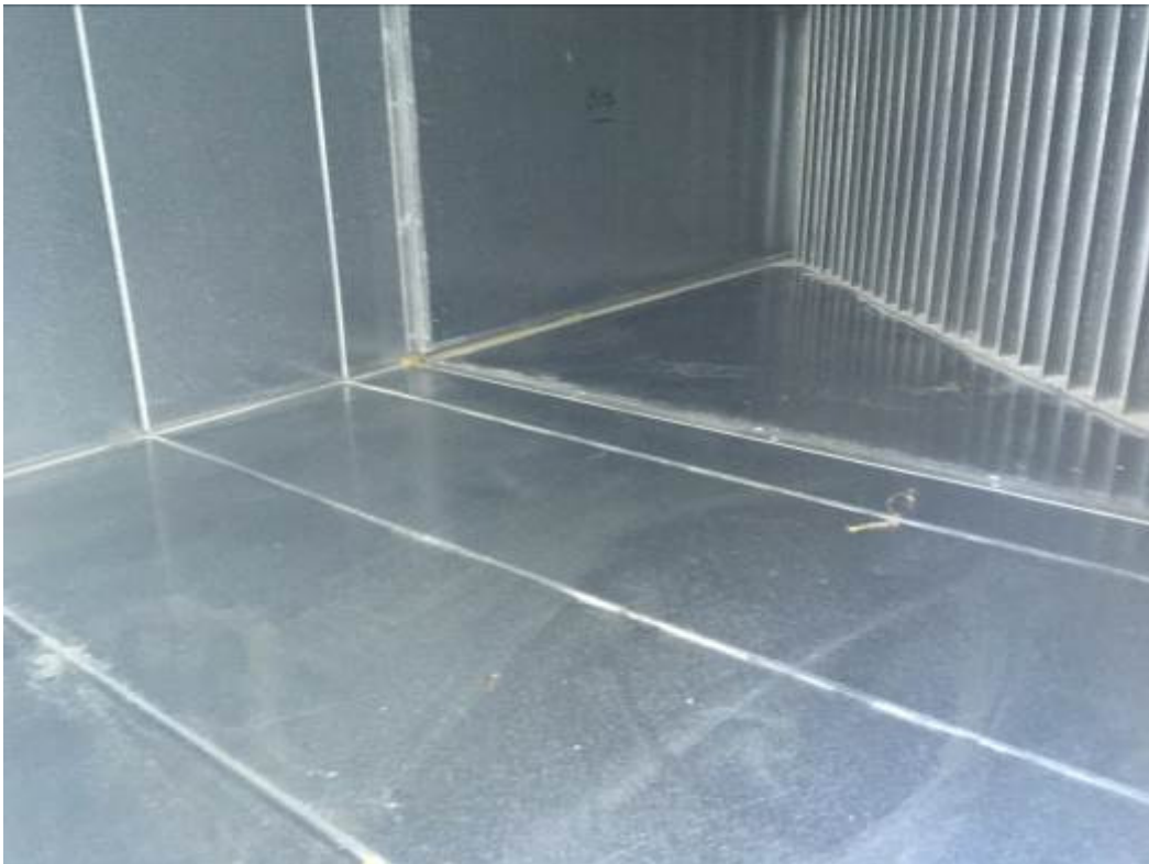
AHU AFTER CLEANING
