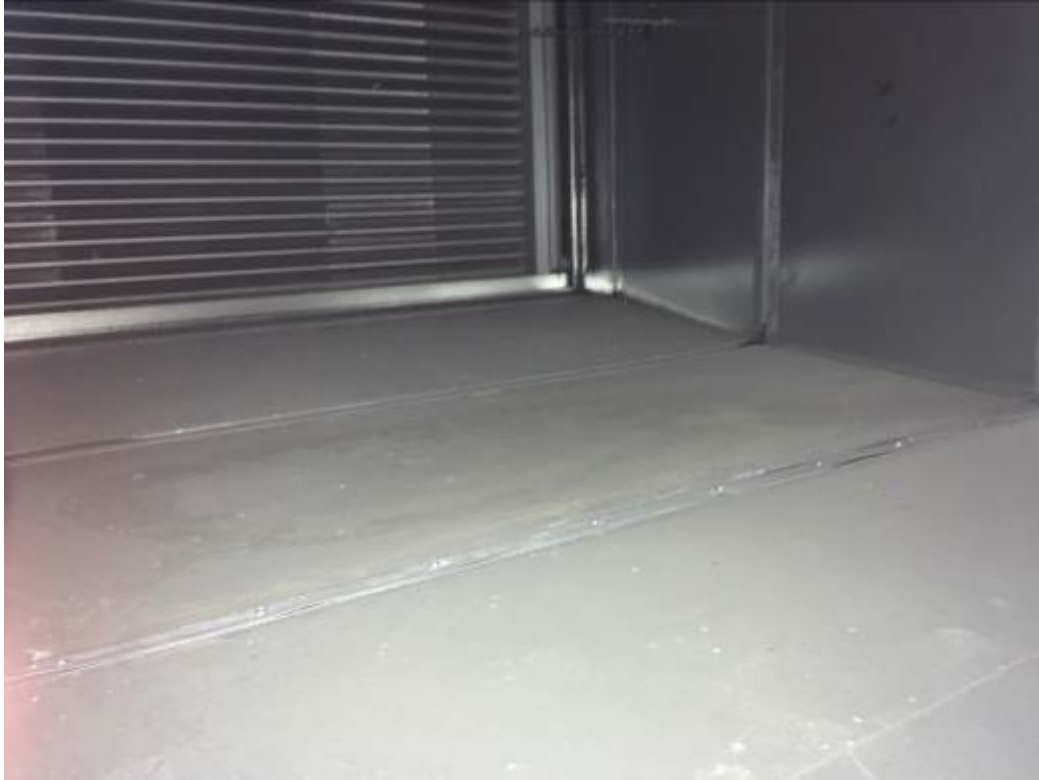
AHU BEFORE CLEANING
