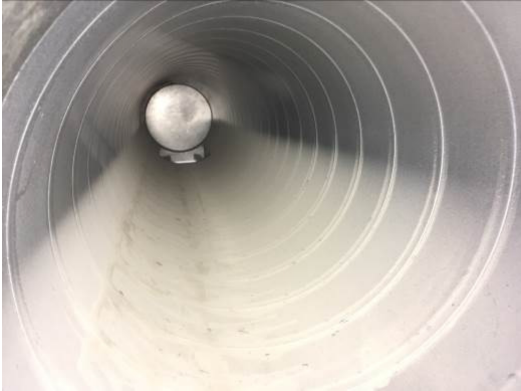
DUCTWORK BEFORE CLEANING
