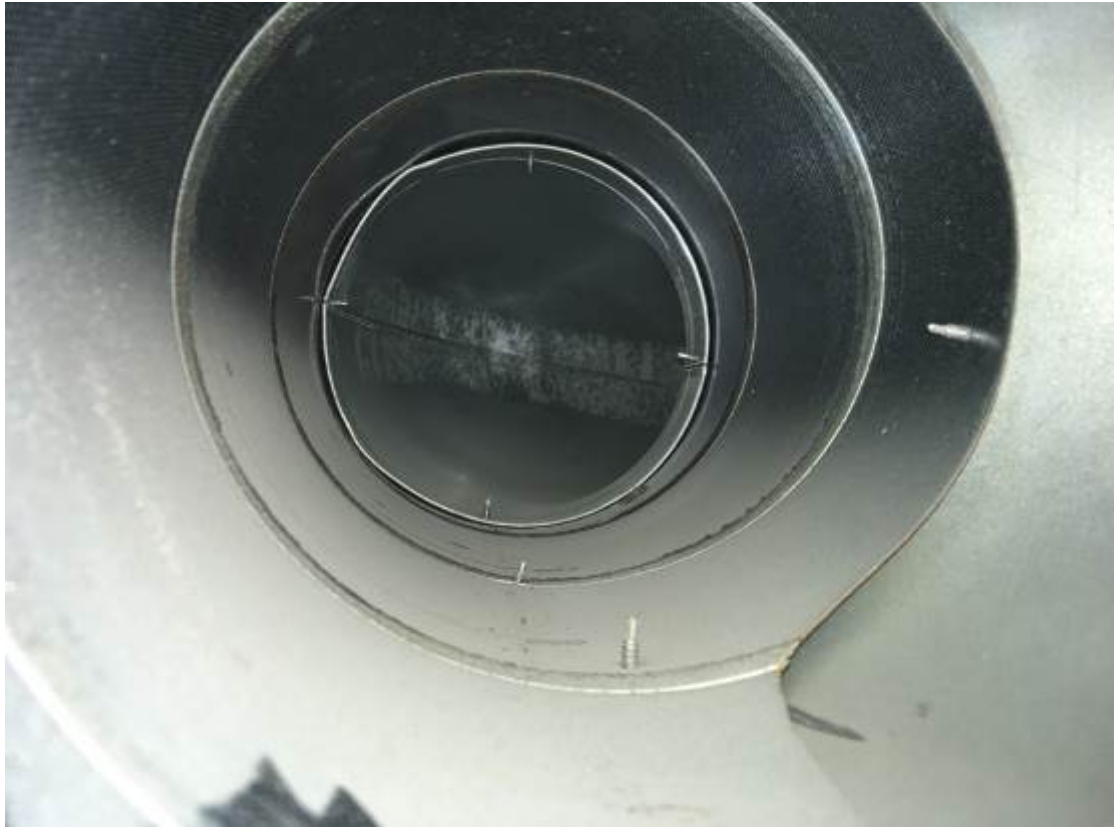
DUCTWORK BEFORE CLEANING
