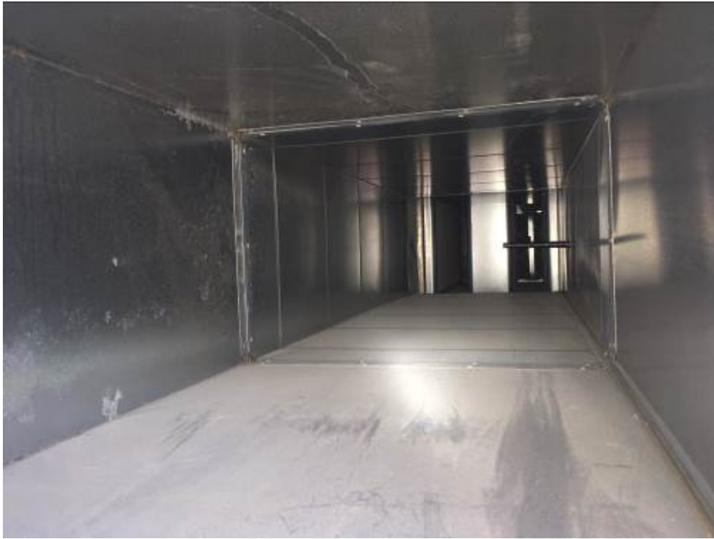
AHU BEFORE CLEANING
