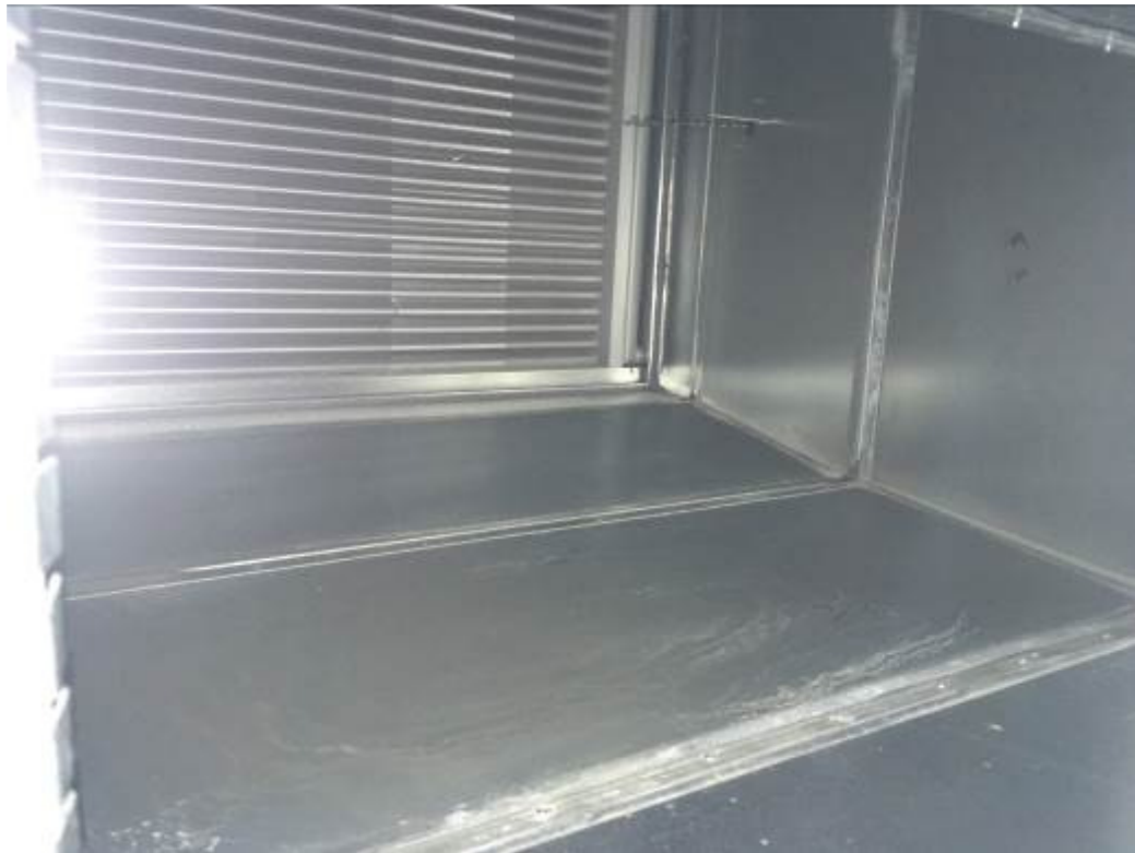
AHU AFTER CLEANING
