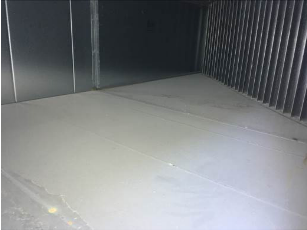
AHU BEFORE CLEANING
