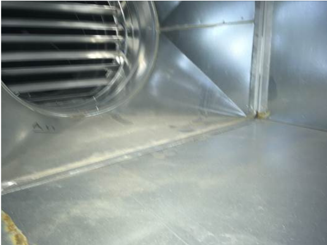
DUCTWORK BEFORE CLEANING
