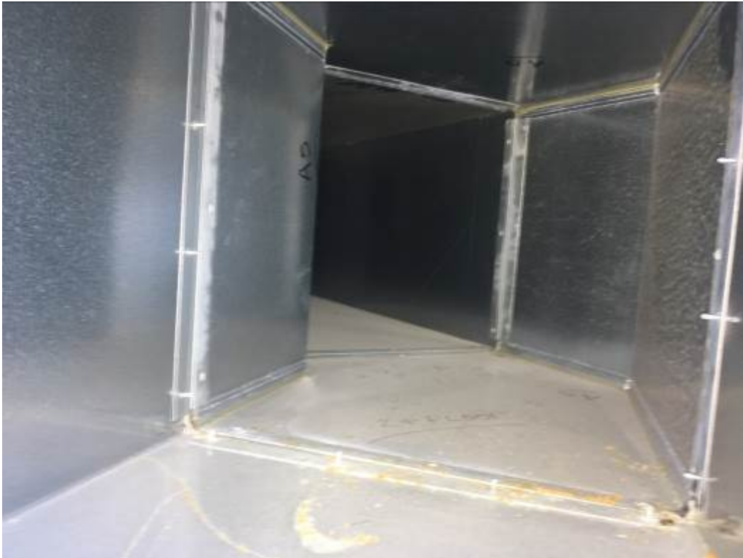
DUCTWORK BEFORE CLEANING
