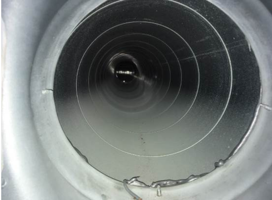
DUCTWORK BEFORE CLEANING
